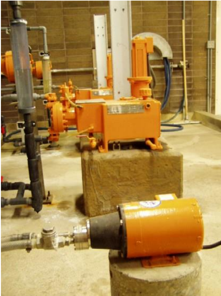
Replaced Pulsafeeder Diaphragm Pump
